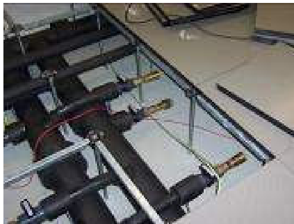
Figure 3: Under floor or overhead piping with quick connects can be added during initial construction, though they can increase construction costs.
